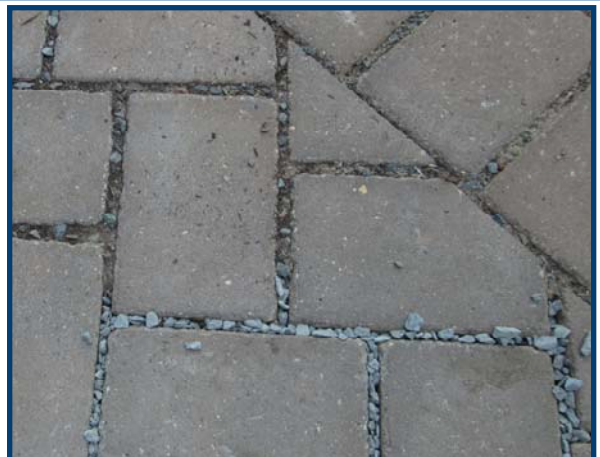
You are done! Notice the difference between the “cleaned” pavers and the clogged pavers.
